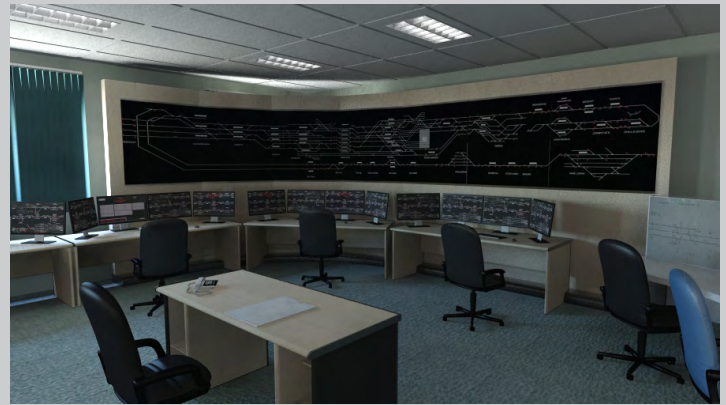
Operation Control Centre
